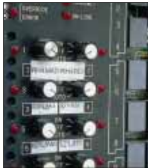
Label switches, relays and other devices
