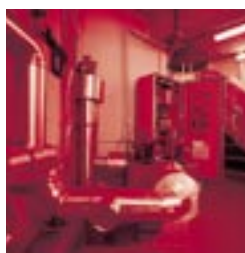
■ Air conditioning units
